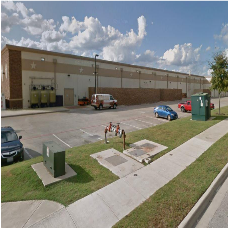
Example of 2 transformers to provide power to multiple locations on the same site (Buc-ee's)
