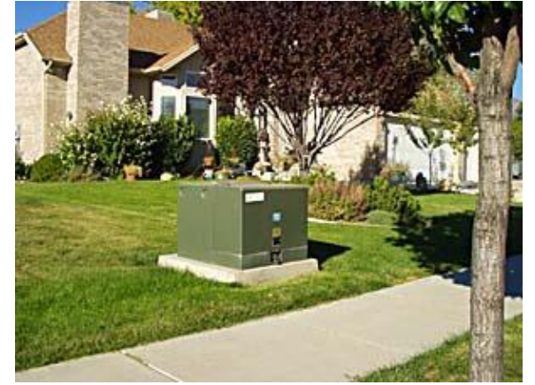
Example of a pad mounted transformer for a residence
