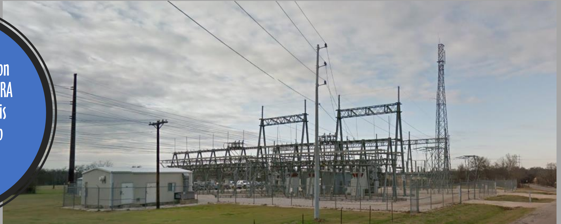
Main Street Sub-Station
